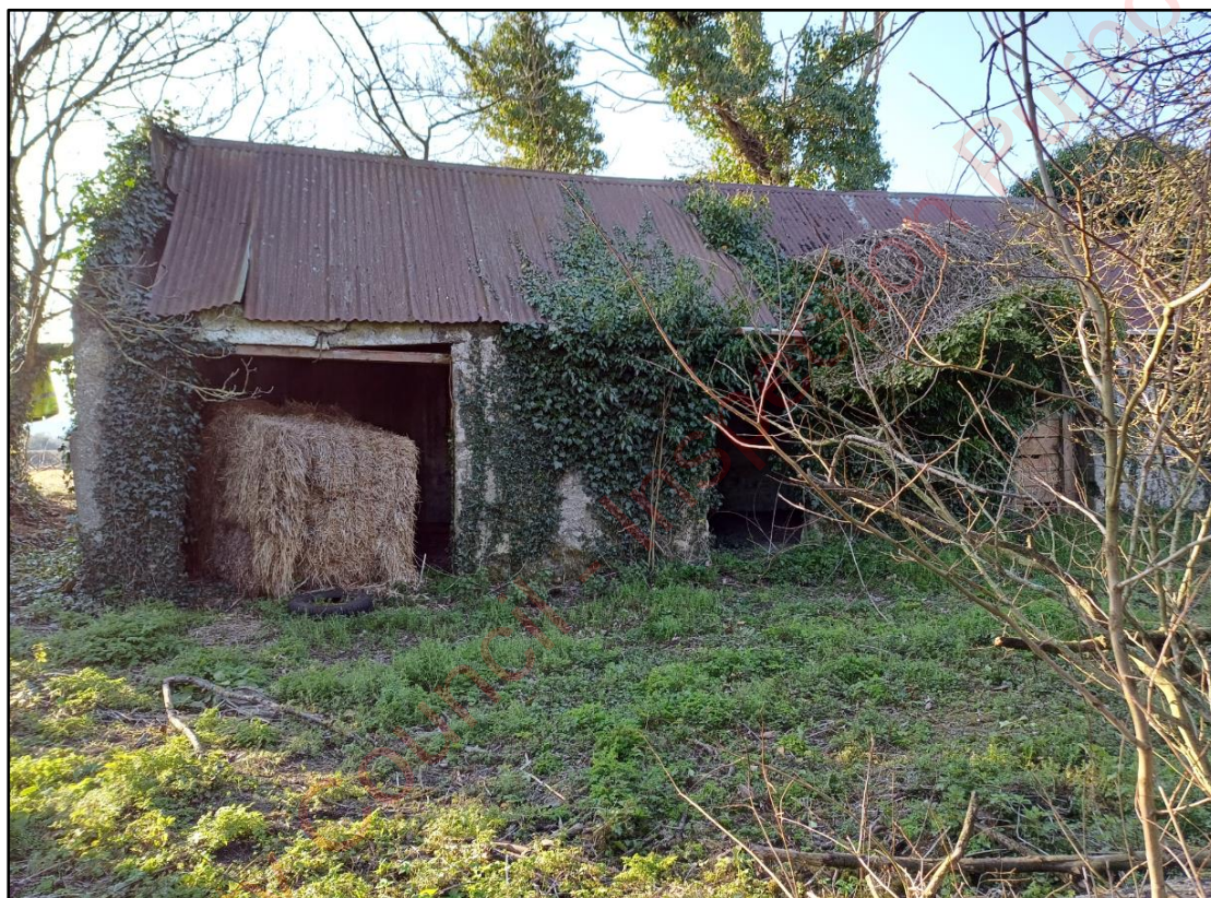
Fig 5: Site inspection photo showing derelict structure on landholding.
